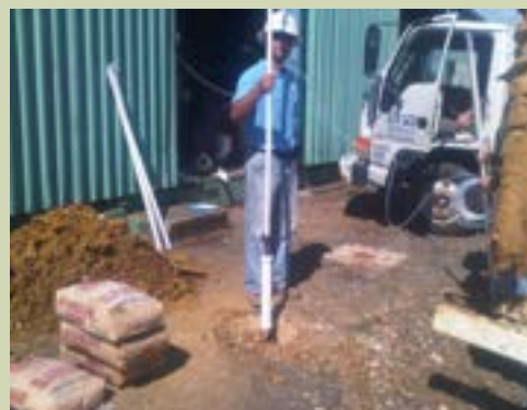
Perozone Injection Wells Project
