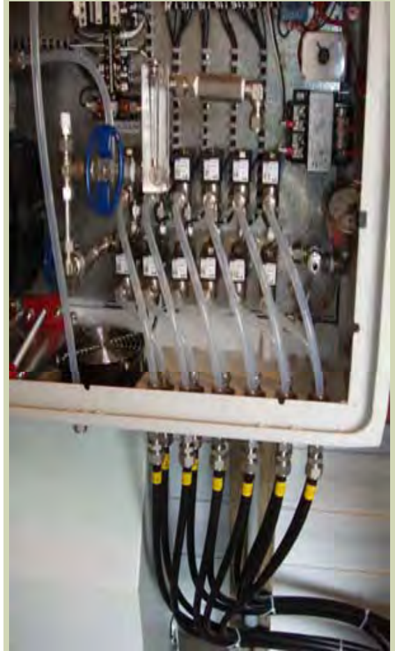
Perozone (Chem-Ox) Injection System
