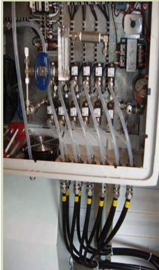
Perozone (Chem-Ox) Injection System
