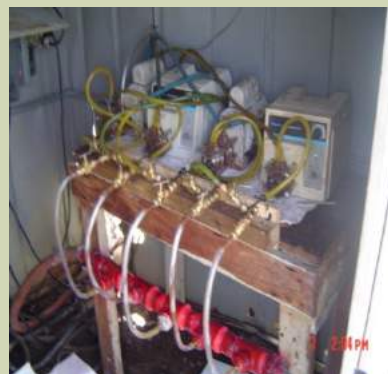
Product Recovery Pump System
