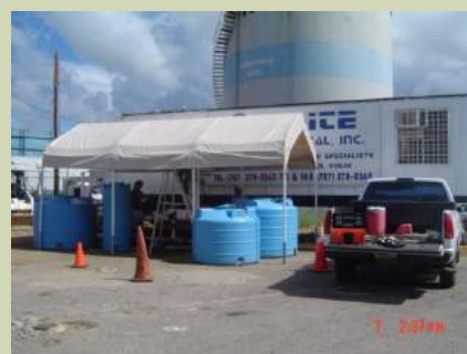
In-Situ Bio-Slurping System
